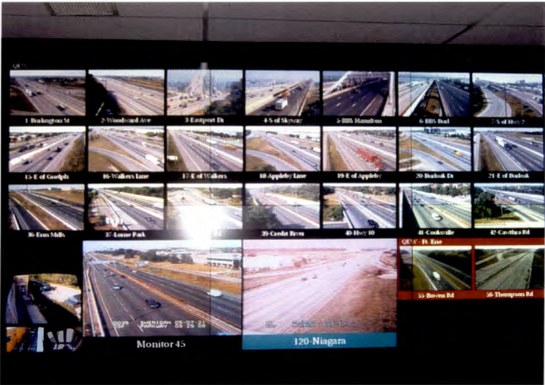
Figure 7-4: Rear Projection Cube Display Wall in Burlington TOC
